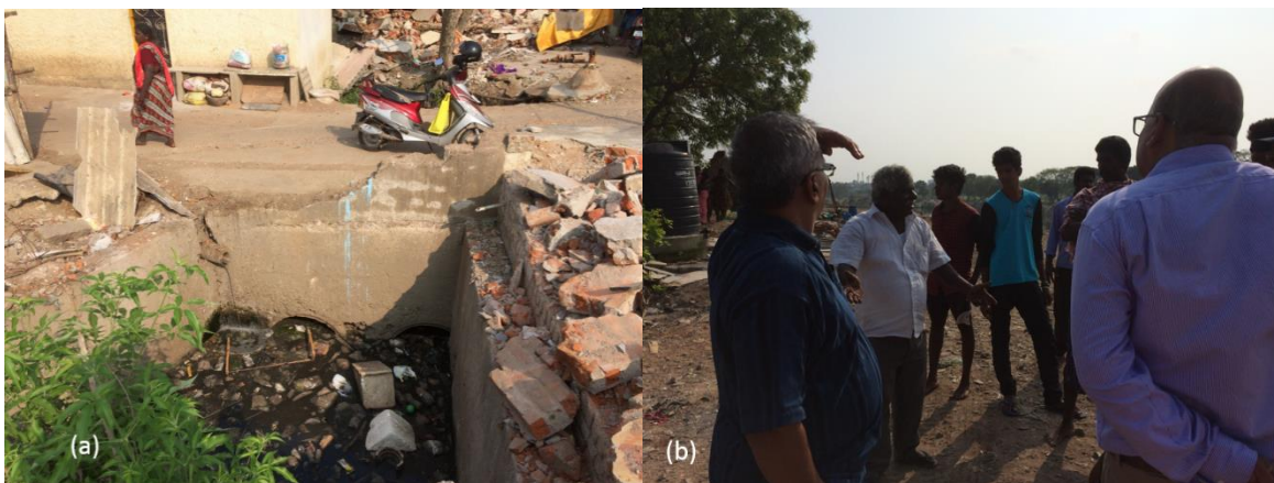
Figure 27: (a) Poor condition of storm water drainage near Adyar River, Ferry Road, (b) Feedback being received from the local residents.
