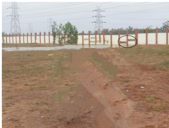
Figure 16: Panels in compound wall taken off to let water flow
