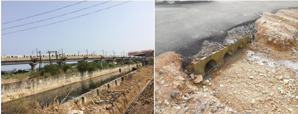
Figure 14: MRTS station on Buckingham Canal Figure 15: Culvert with inadequate Capacity
