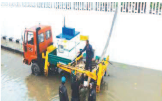
Pump set deployed in subways
